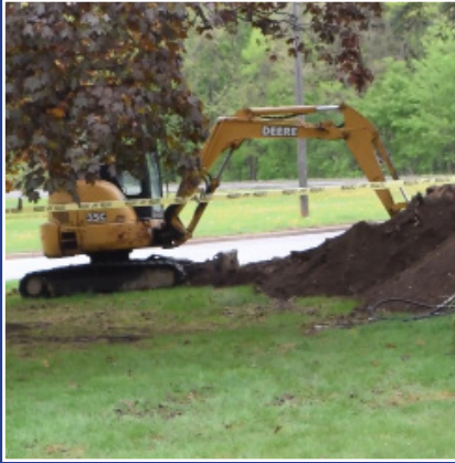
1. The area around the site is excavated to the bottom of the footing.
